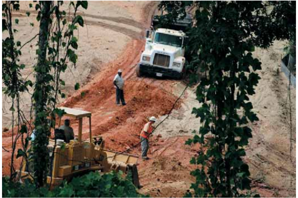
Construction is underway on Aug. 20 as workers clear land for the new Faith Newton Hobson Chapel on Wesleyan Drive on Southern Wesleyan University's campus in Central.
